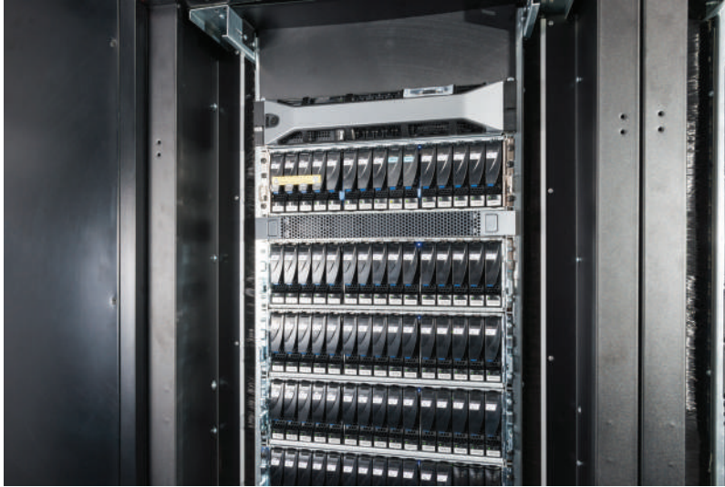
Figure 11.14 A storage array.
